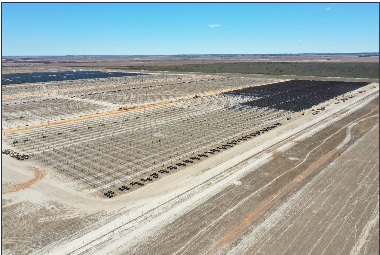
New stage 2 solar panels mounted on their tracking systems with stage 1 panels visible in the distance
