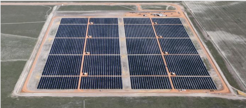
The 150,000 solar PV panels of stage one with the second stage to be developed...
