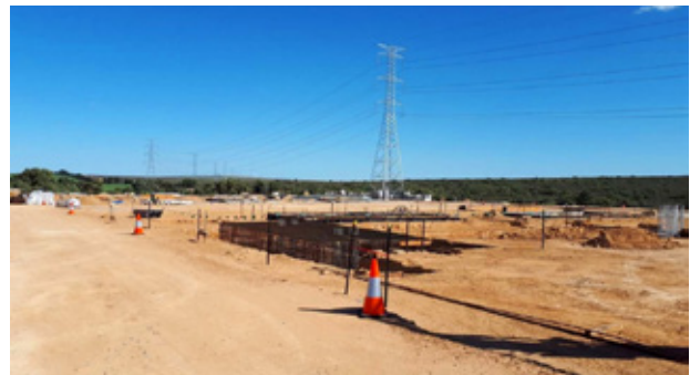
Pictured: Eneabba Terminal under construction by Western Power to connect Warradarge wind farm to the 330kV grid.
