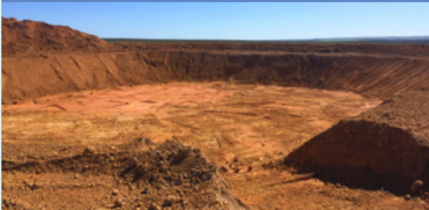
Pictured: An excavation for one of the wind turbine foundations at Warradarge wind farm which measure up to 20m wide and 3m deep.
